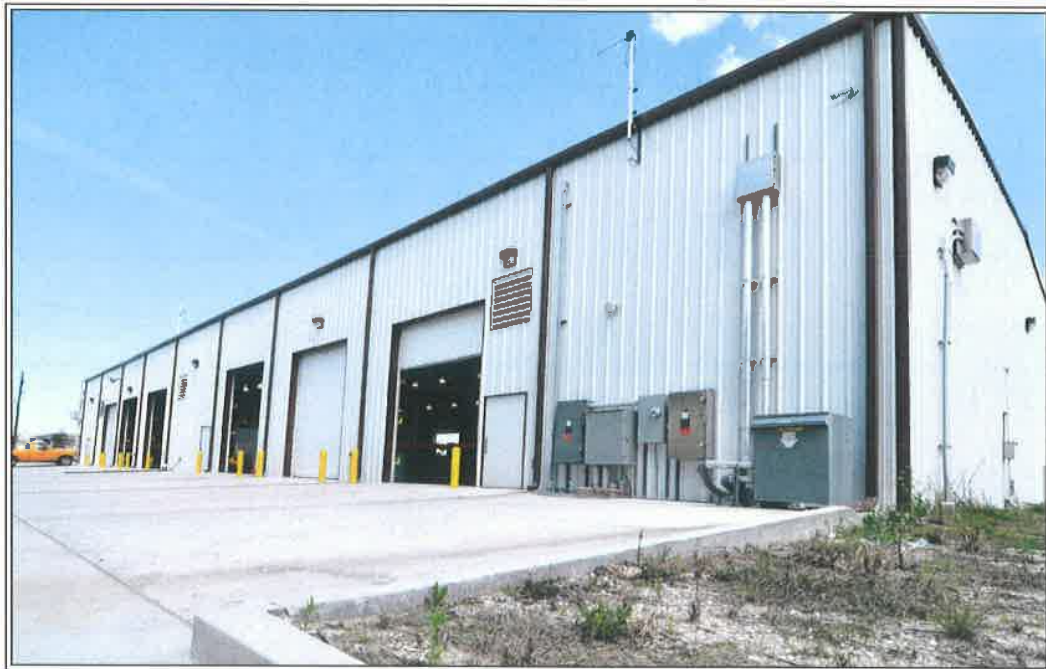
The vehicle and equipment repair and service garages at Central Yard are being repaired and constructed. These facilities are critical to operations. Thus, FEMA funded a facility to serve as an interim location to service light and large vehicles and heavy equipment. This new facility is a temporary location while Garages I and II repairs and construction is completed. It houses personnel and equipment needed to service the vehicle fleet and equipment. It is called a site relocation facility. The FEMA funding for the project was $1.8 million. Upon completion, the new garage will be the home of the body shop. Besides the garages, Central Yard is the service facility of the board. The site, also, includes support services, networks, meter reading, environmental affairs and the warehouse.
